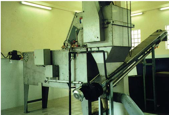
The ROTOPRESS® compactor at a Combi-Guard® outlet operating faecal sludge.
